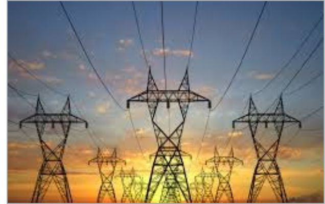
Power In The Network
